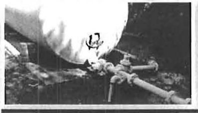
Hydro storage tank
