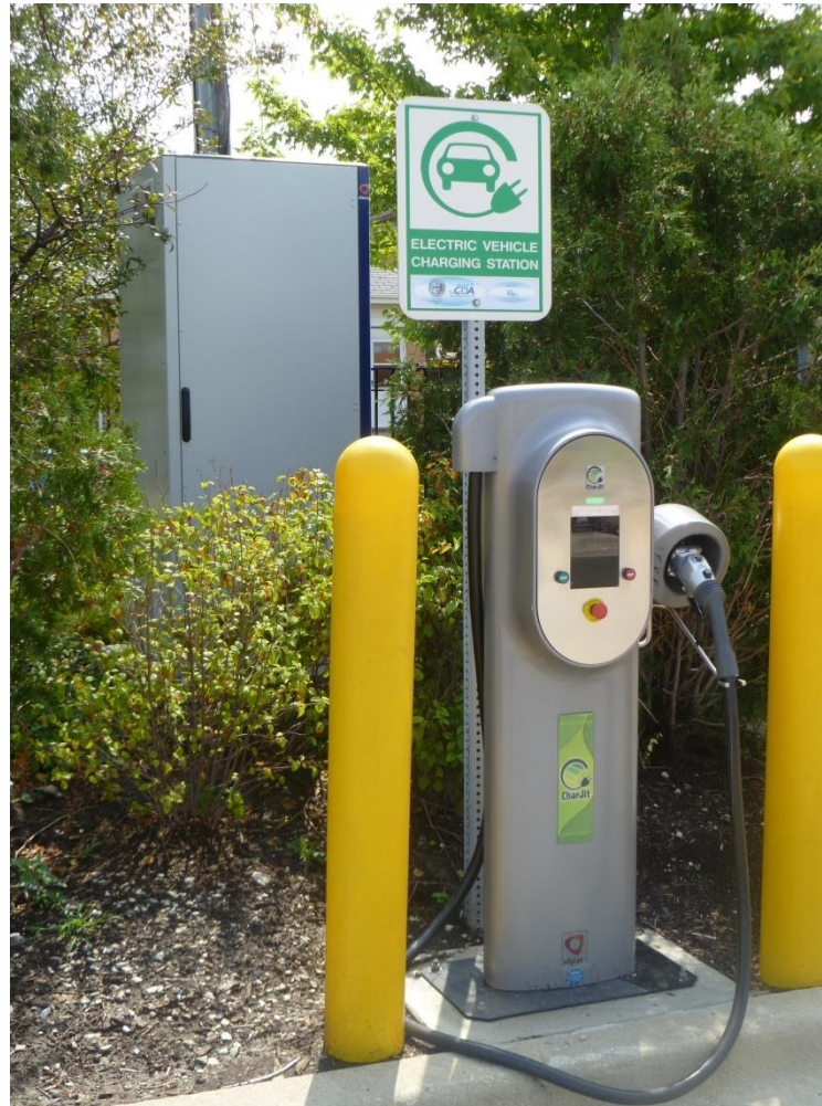
Power cabinet in the back Central controller and user interface in the front
