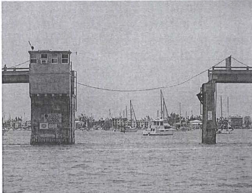
OPENING OF 20TH STREET BRIDGE WHERE POWER LINE WAS POST-COLLISION
