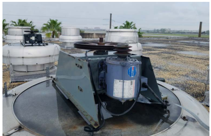
Watkins Substation – Roof Exhaust Fan
