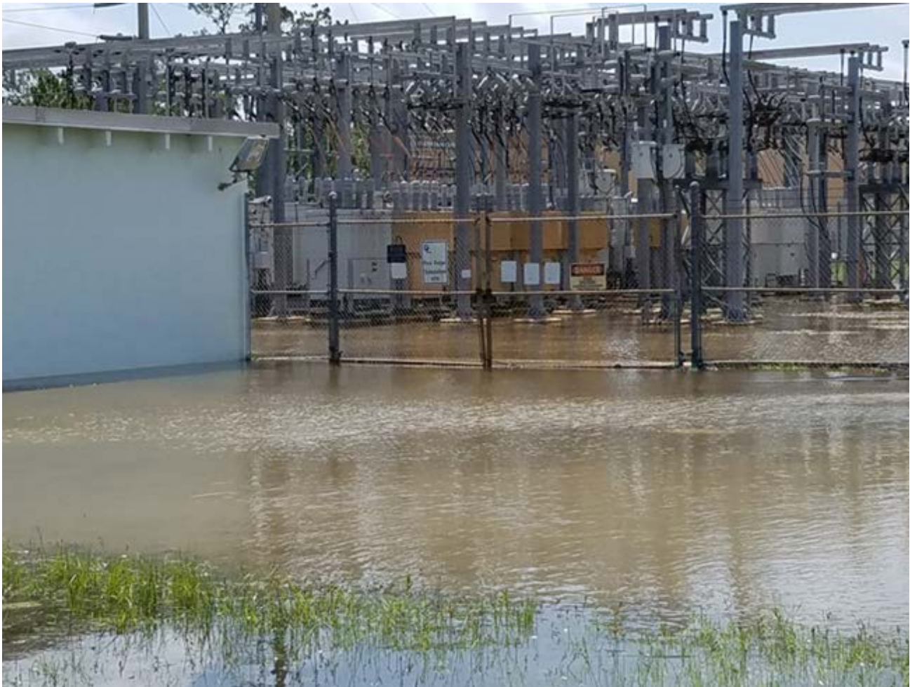
Pine Ridge Substation rain event flooding
