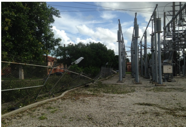
Crystal River Substation – Fence
