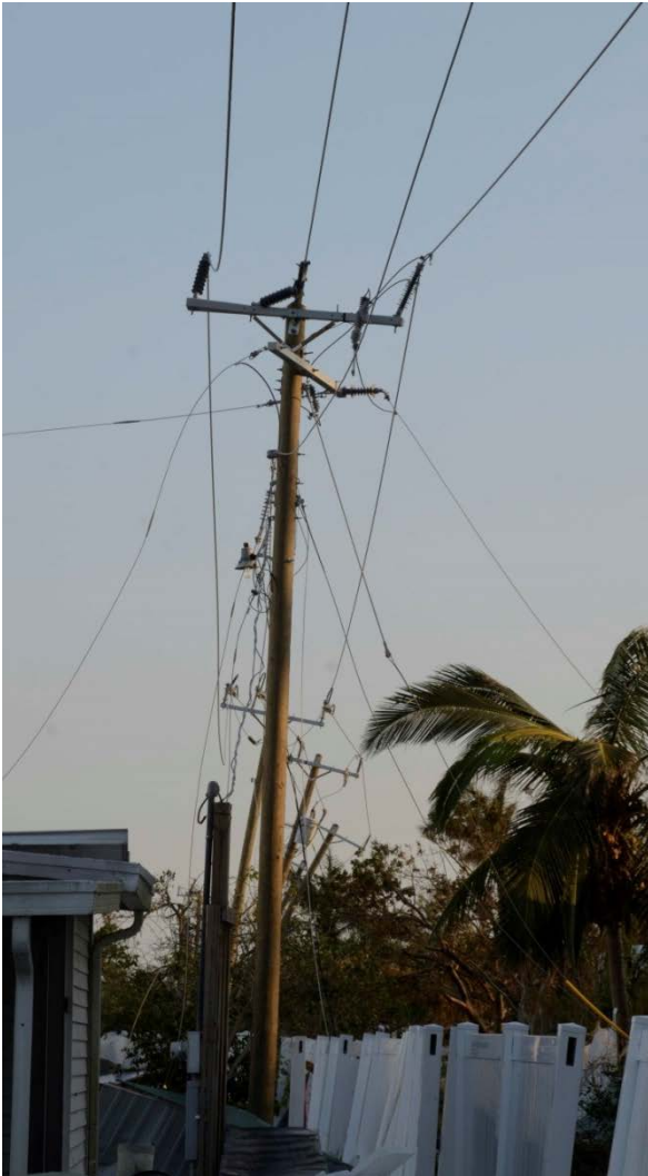
View of leaning poles
