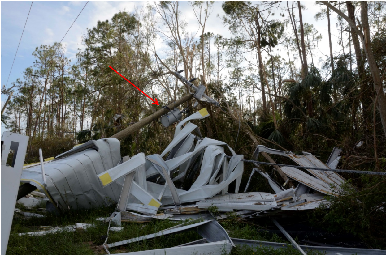
Pole down with transformer in West area due to trailer park debris
