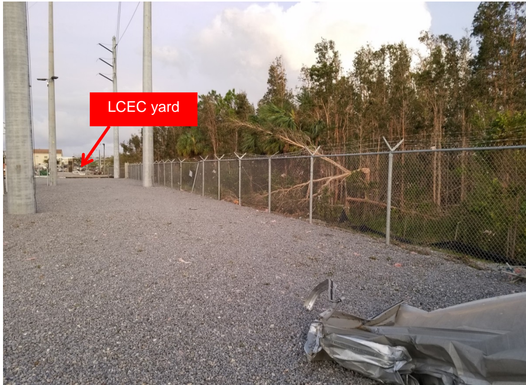
Belle Meade Substation (Looking East)
