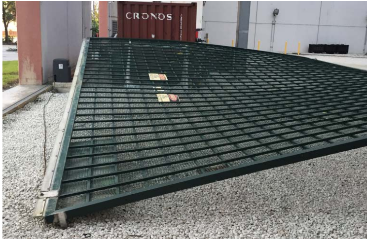
Natural Bridge Substation – Gate
