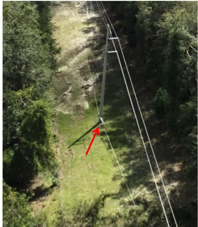
Structure 55R13A – Broken insulator
