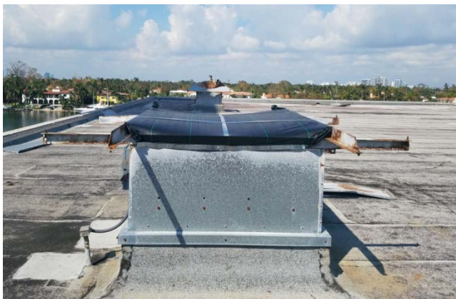
Indian Creek Substation – Roof Exhaust Fan
