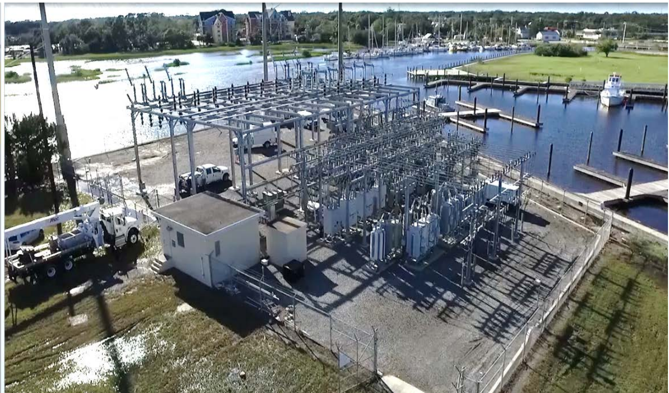
St. Augustine Substation
