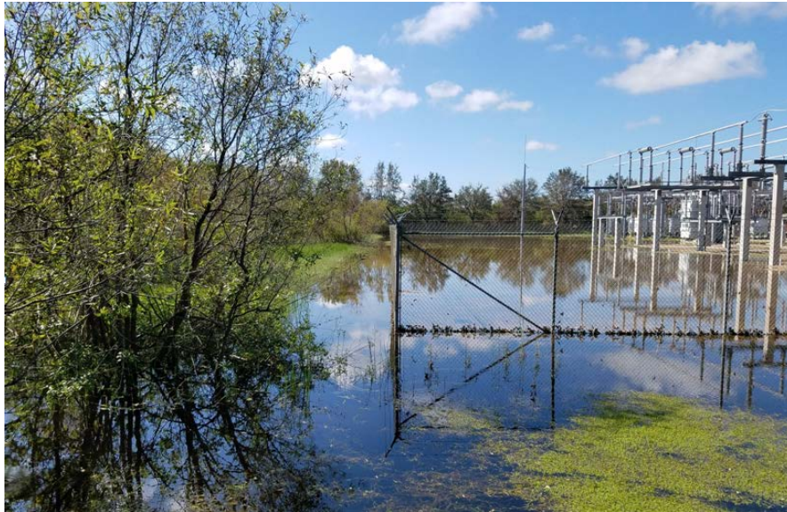
Corkscrew Substation Rain Event Flooding
