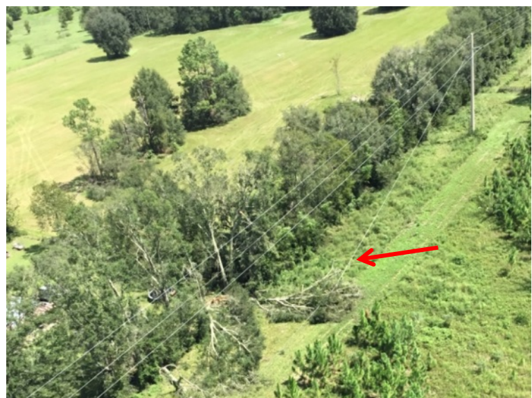
Structure 112R1 - Wire down due to vegetation
