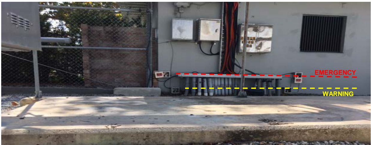
Alarm log for South Daytona Substation
