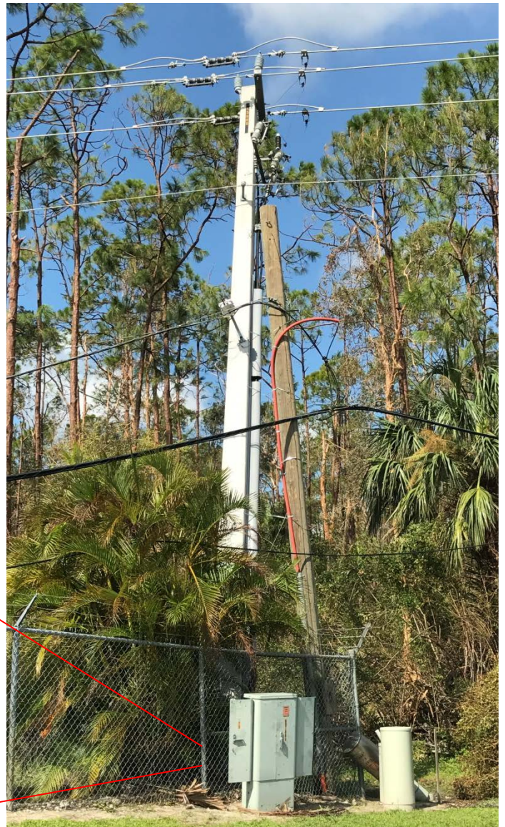
Leaning concrete pole
