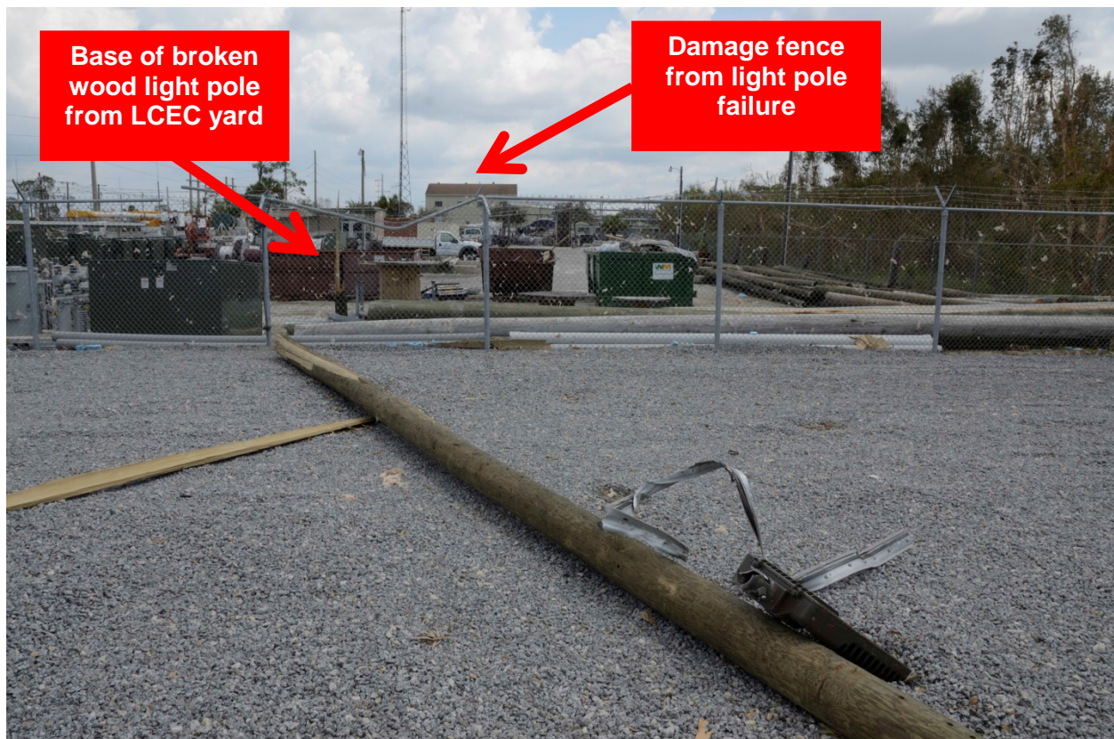
Belle Meade Substation (Looking East) adjacent to LCEC yard (Lee County Electric Coop)
