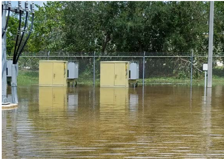
Pine Ridge Substation Flooding
