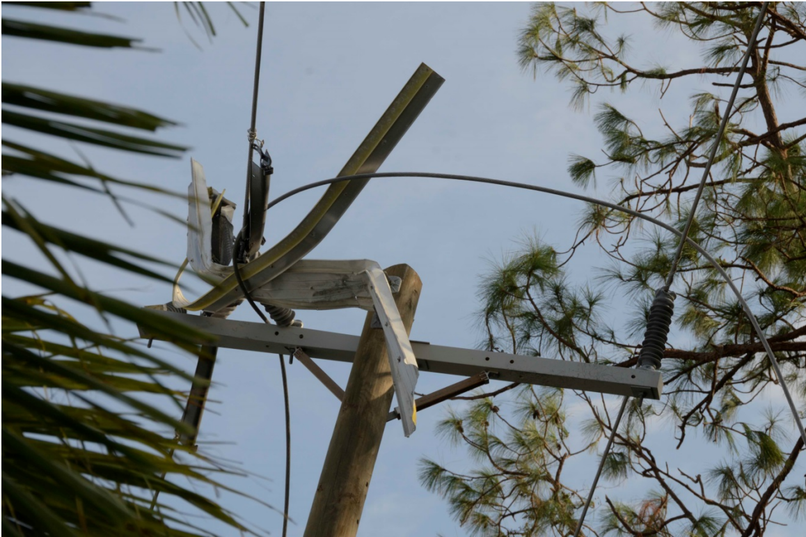
Debris wrapped around pole in line.
