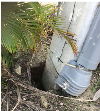
Base of leaning concrete pole
