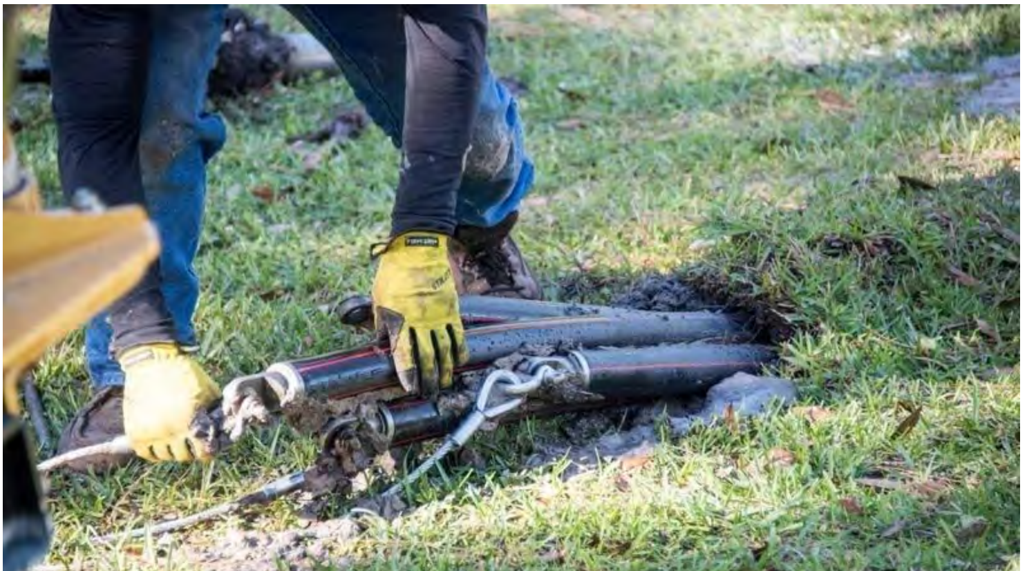
A worker for FPL burys a power line in a neighborhood. (SSMG)
