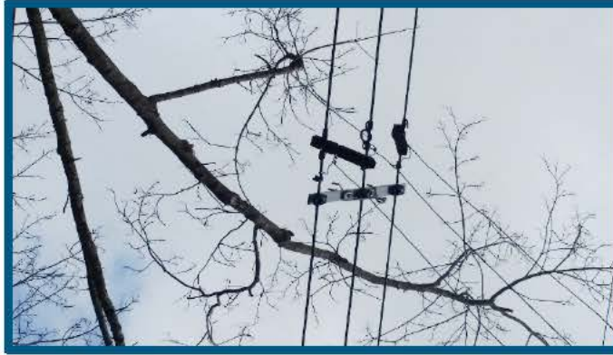
Figure 4: Three examples of open wire secondary that will be addressed
