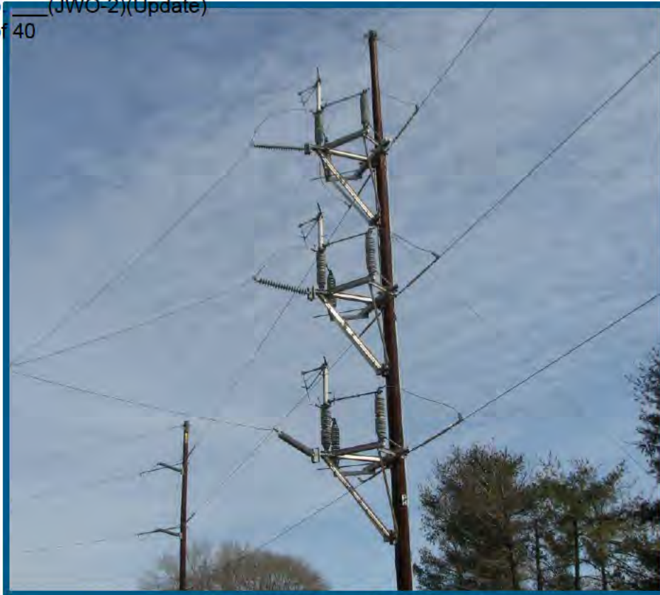
Figure 3: DEF Manually Operated Switch
