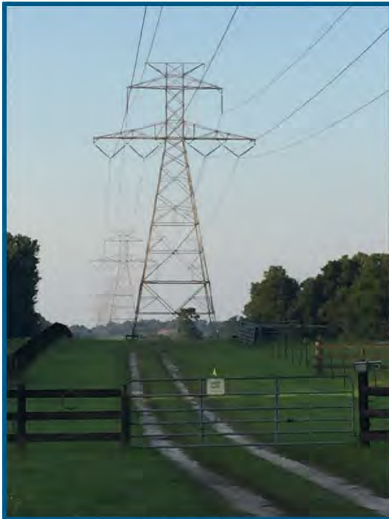
Figure 2: Double Circuit Tower
