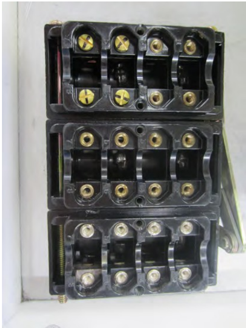
Front of Auxiliary Switches
