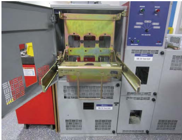
Breaker Frame on Test Cell Rails
