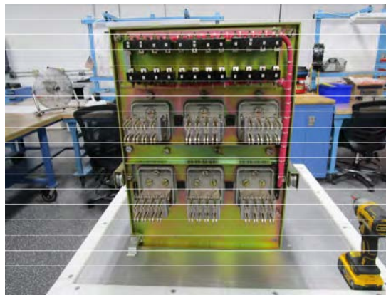
As Received Rear of Breaker
