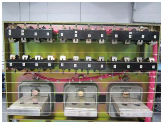
Secondary Contact Assembly on Breaker
