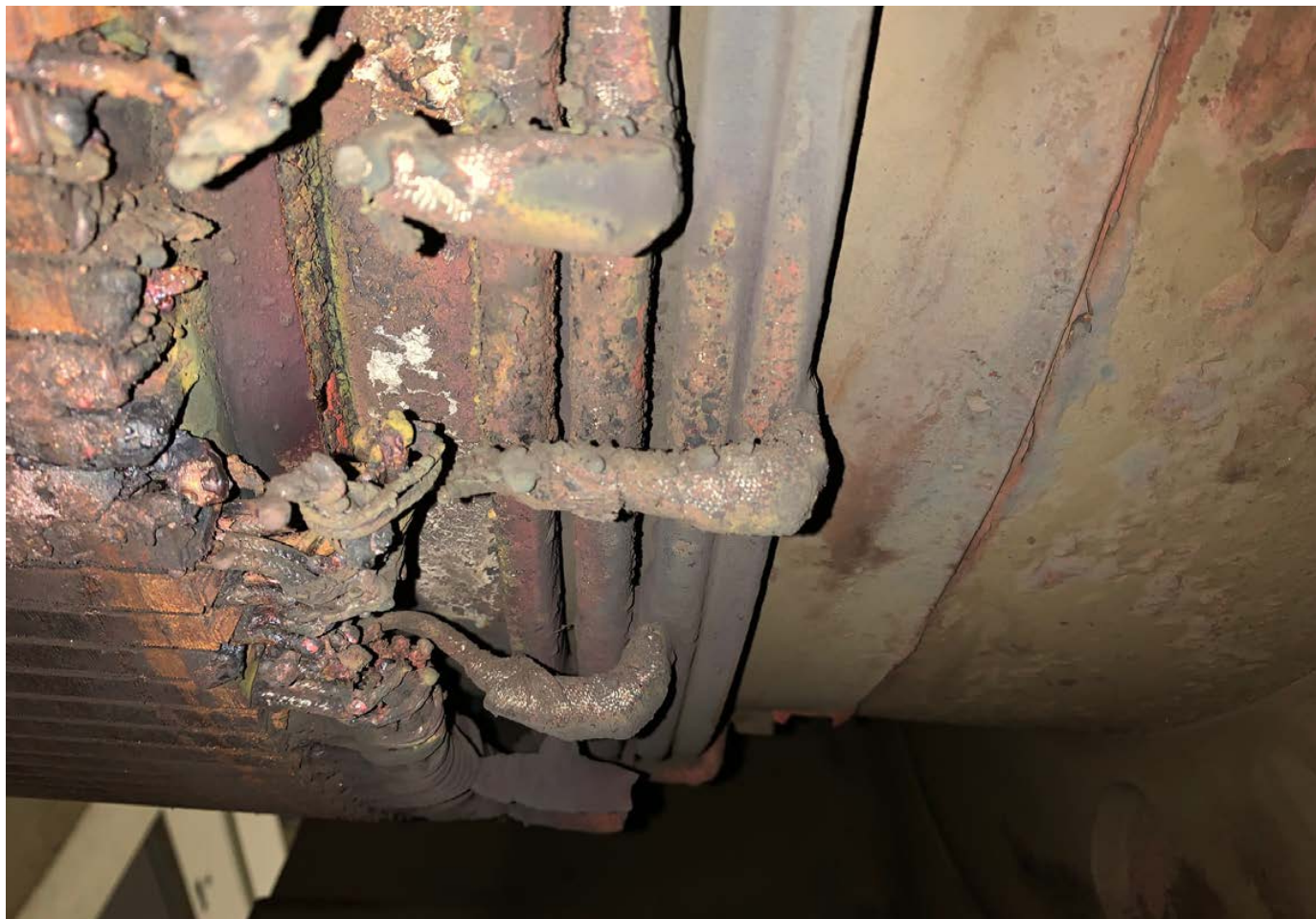
Fig. 7 PMG Stator Coil Connection Ring Failures
