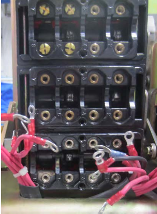
Front of Auxiliary Switches
