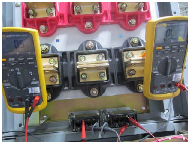
Switch Monitoring Shows a Change of State
