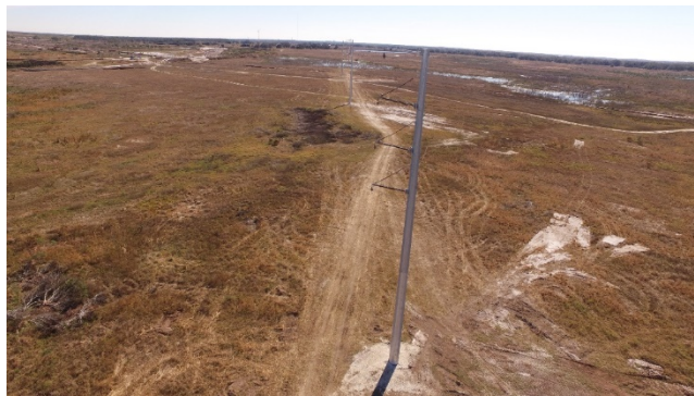
Completed steel structure with insulators
