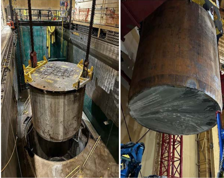
Top Package in Storage, Final Insulation Removal, Completed RV Bottom Horizontal Pre-Cut
