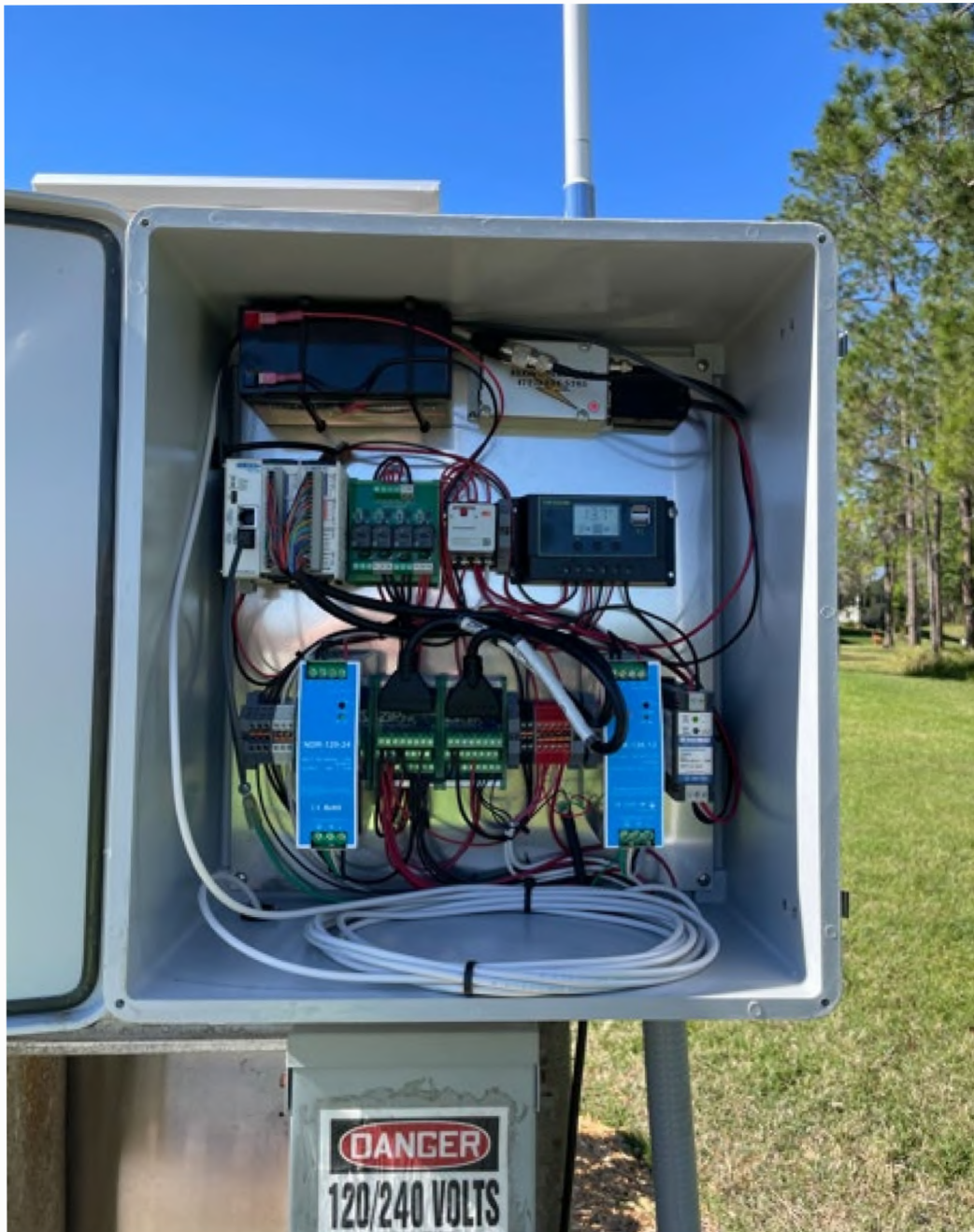
Lift Station #6B
