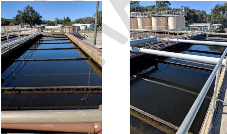
Figure 4: Clarifier North Train (left) and South Train (right)
