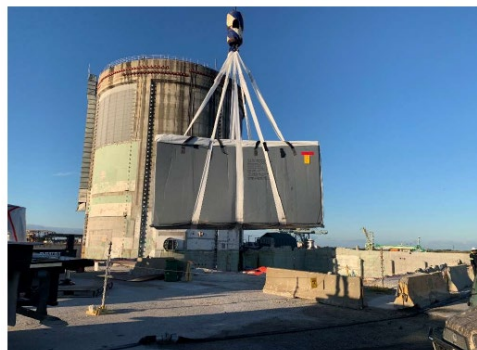
Substructure Bag Loadout
