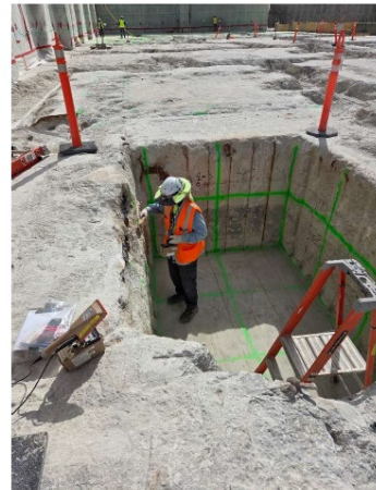
FSS Laundry and Shower Sump
