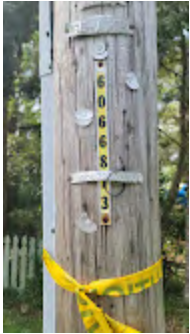
POLE WITH RISER.jpg 2914K
