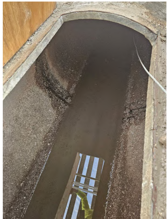
Raw Water Discharge Pipe Opening
