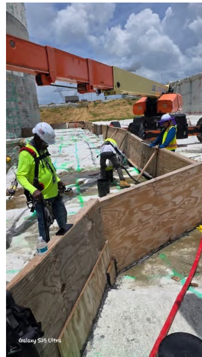
FSS Seawater Room
