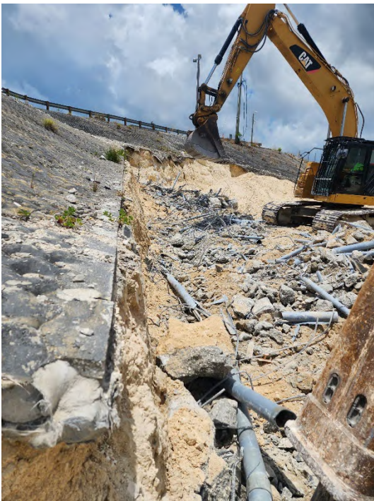
TSC Duct Bank
