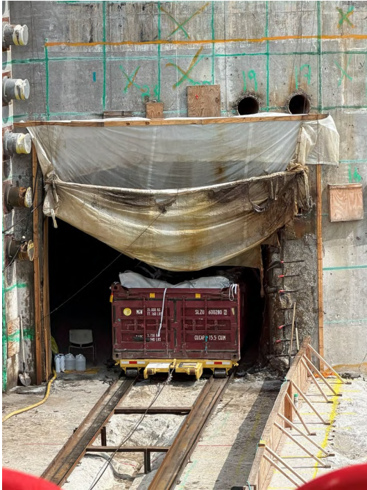
Reactor Building Loadout
