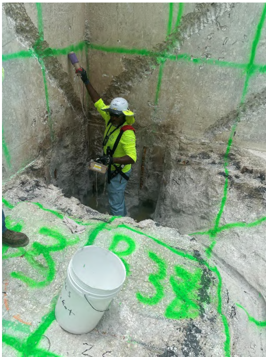
FSS Decay Heat Vault Sump
