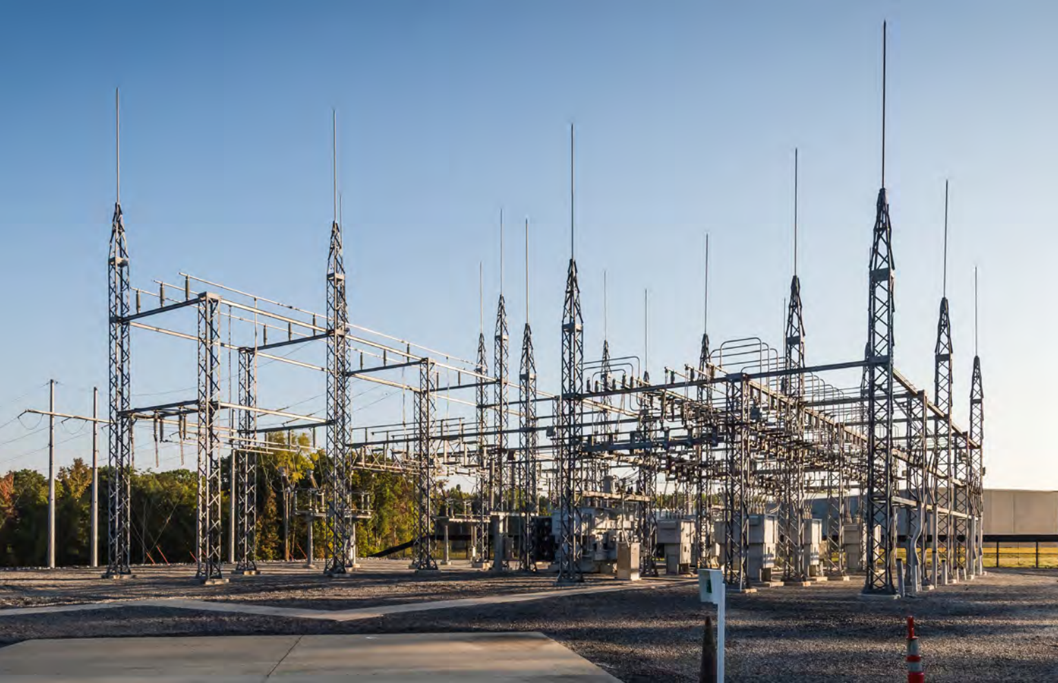
Self Healing Grid Substation
